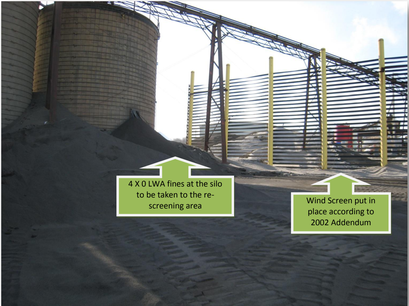
Figure 2. The 4 X 0 LWA fines are stored at the silo located at the southeast portion of the facility just south of Kiln 1. To minimize dust generation, a 50 % porosity wind screen was installed as part of the 2002 Fugitive Plan Addendum.
